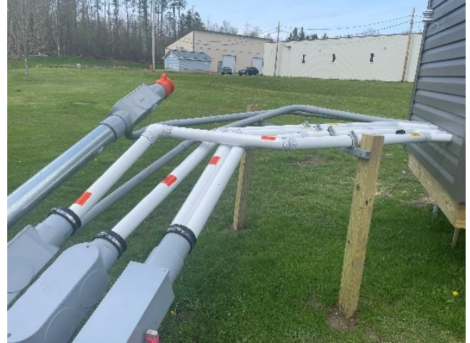
Pictured above are the instrument and sample conduits exiting the rear of the station, which enter the creek via a series of pipes.
