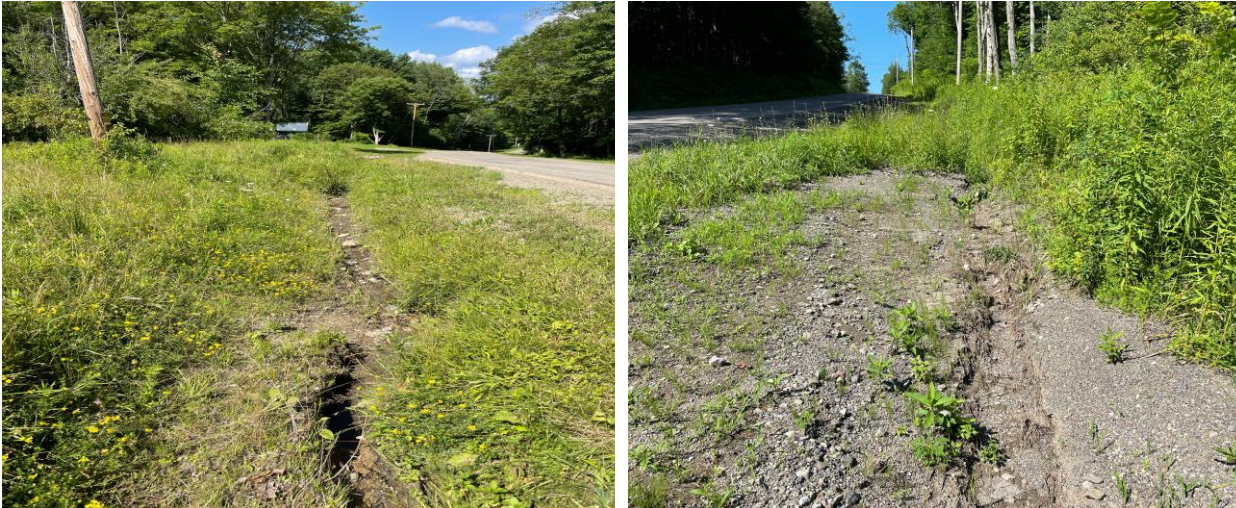
Above: Erosion paths can be seen along the north bank of Moore road, left, and the east side of Burdick road, right.
